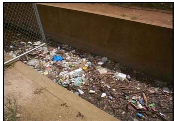
Trash in a Wai’anae drainage canal.
